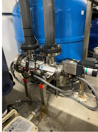
*Aquatic Center - Pool UV System
