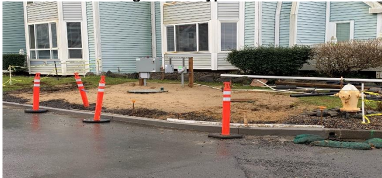
New Pump Station
