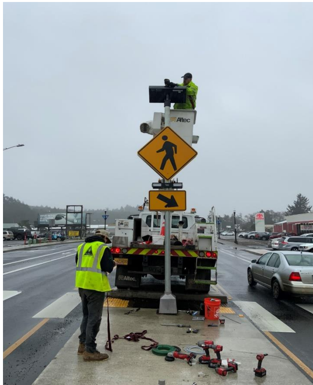
Hwy. 101 Center Median Flashing Beacon
