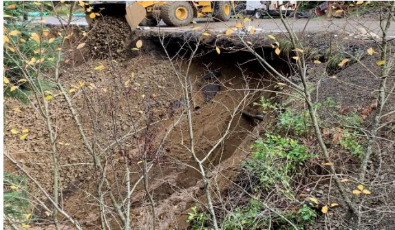
Broken 8" Sewer Pipe at 2 nd Slide
