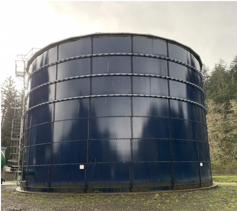
Water Treatment Plan 450,000 Creswell Water Tank
