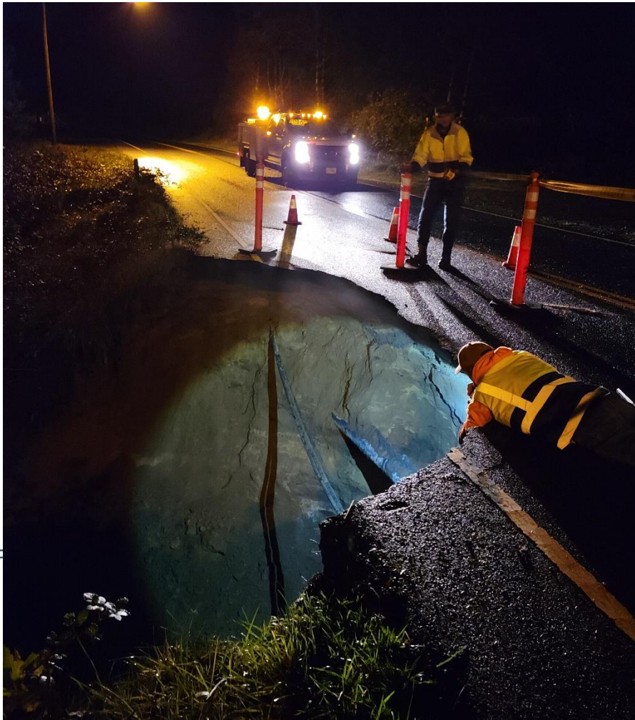
Oceanview Drive Storm Water Emergency
