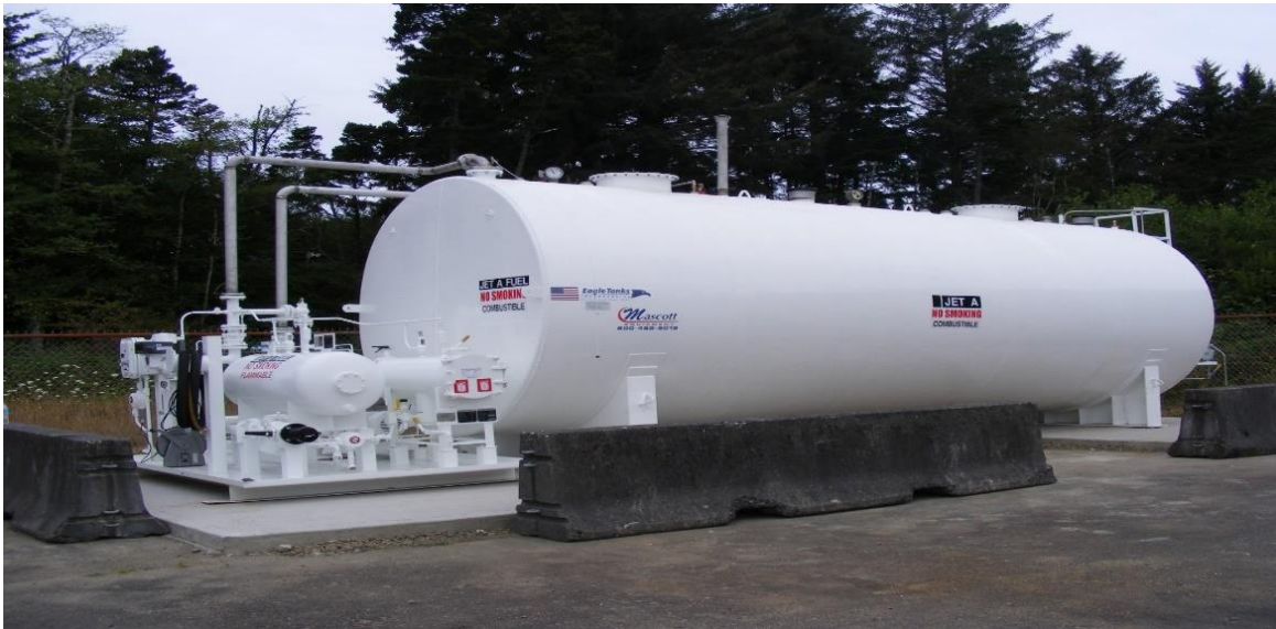
Jet A 12000 Gallon Fuel Tank- Airport
