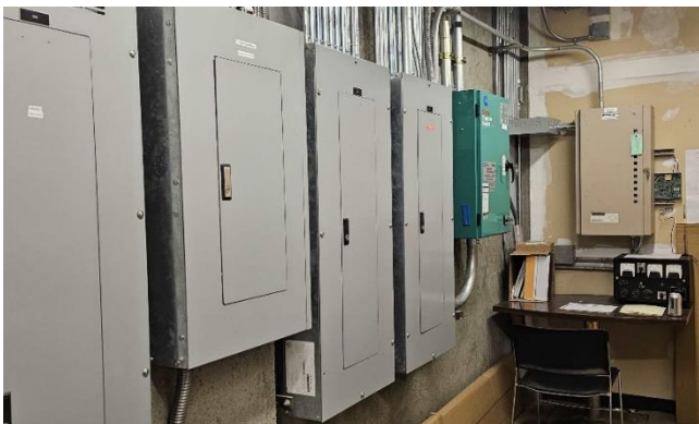
City Hall Electrical Panel
