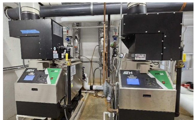
Aquatic Center Boilers
