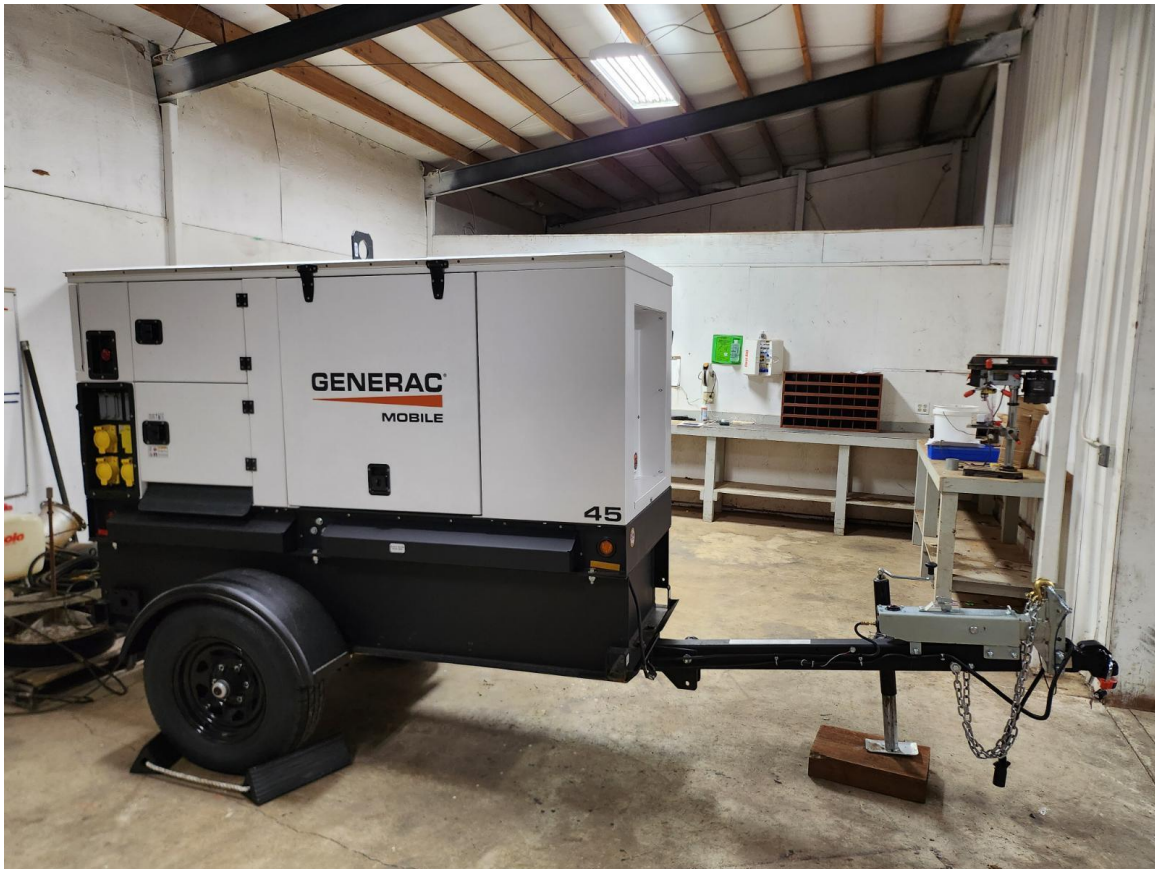
Mobile Generator for the Wastewater Treatment Plant
