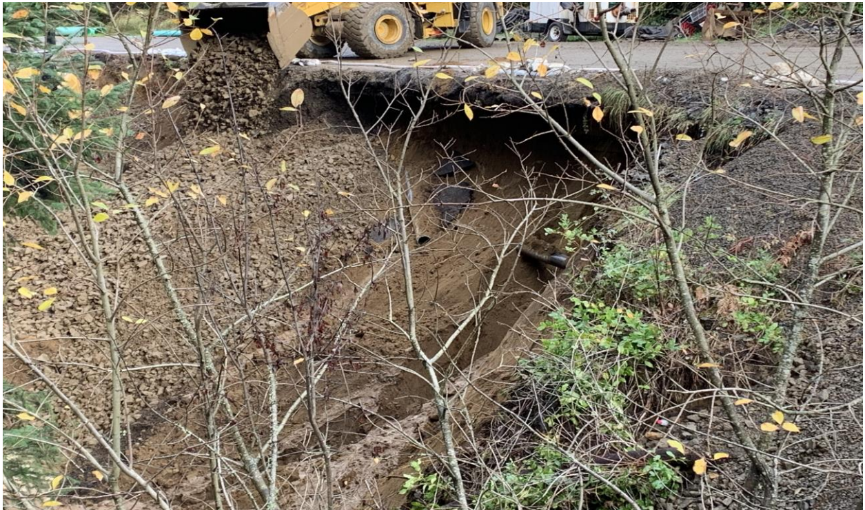
Broken 8" Sewer Pipe at 2 nd Slide
