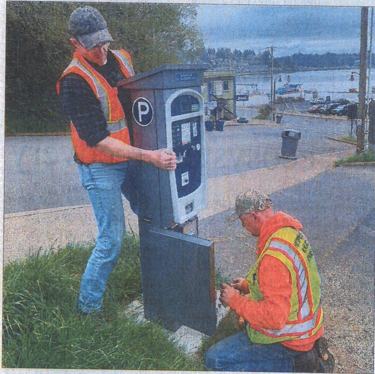
Travis Tibbetts, standing, and Matt Hall, with the Newport Public Works Department, install a pay station at the Fall Street parking lot. It is one of 10 stations that will be located throughout the Bayfront. (Photo by Steve Card)
