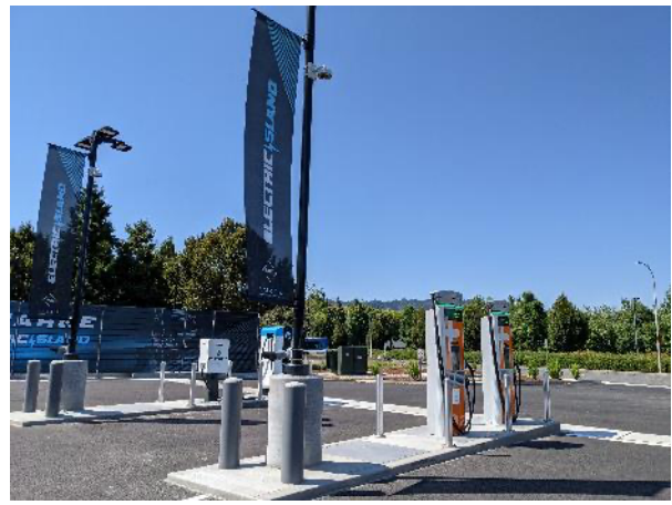
Electric Island charging hub (Swan Island, Portland, OR)
