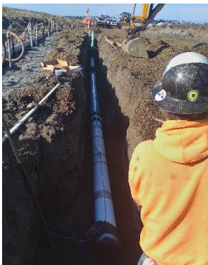
Yaquina Industrial Park Waterline
