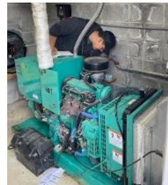
WWC crew checking lift station generators
