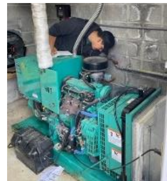
Collections Crew Checking Lift Station Generator
