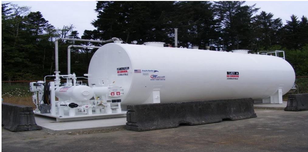
Jet A 12000 Gallon Fuel Tank- Airport
