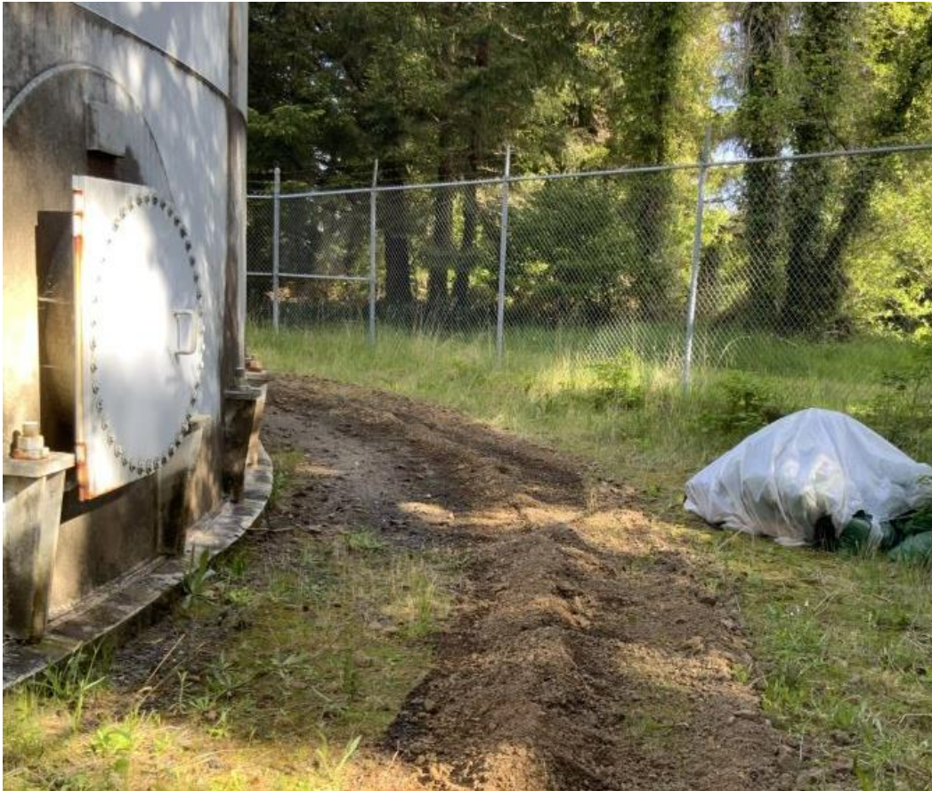
Cathodic Protection at Yaquina Heights Tank
