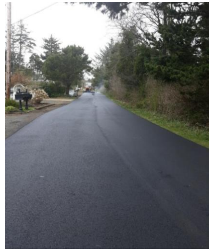
NE Megginson Street After Skin Patch
