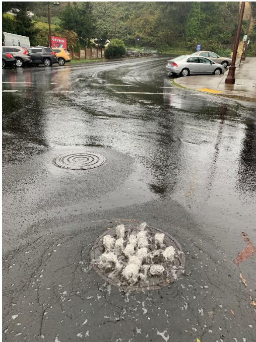
Failed Storm on the Bayfront
