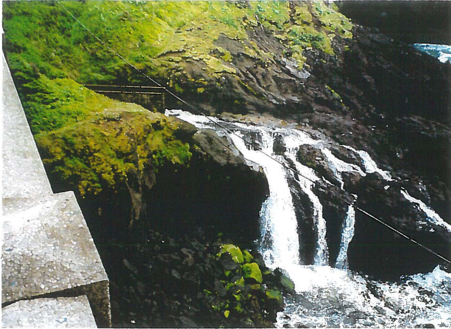
Photograph of 30- to 40-foot plunge where Rocky Creek discharges to the ocean. The concrete flume is an extension of the Highway 101 culvert.
